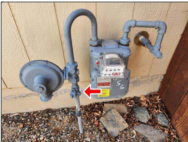
5.11 Item 1(Picture) main fuel shut-off valve
