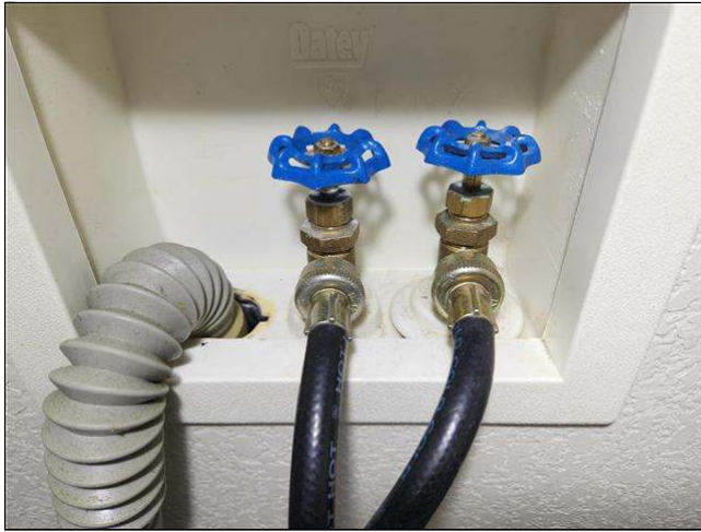
5.6 Item 1(Picture) laundry hook-ups
