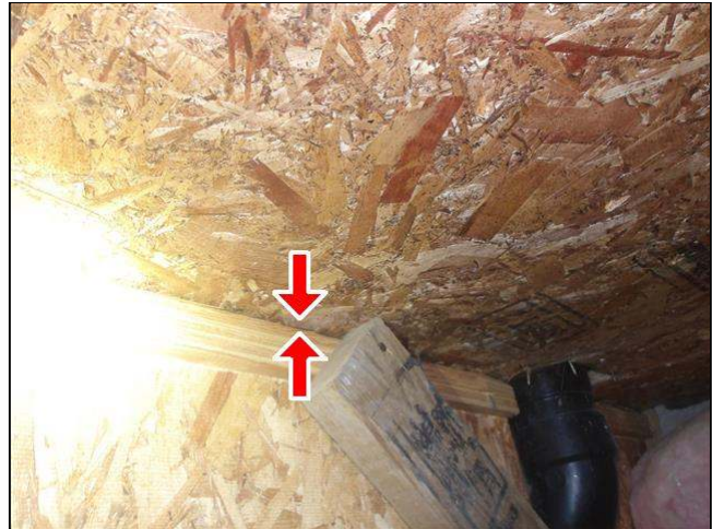
3.6 Item 2(Picture) causing it to come loose from the floor joist
