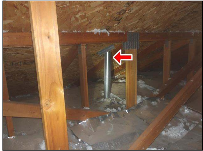
9.4 Item 2(Picture) properly ducted to the exterior
