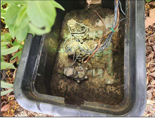
5.13 Item 1(Picture) irrigation box/valves
