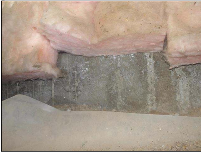
1.7 Item 1(Picture) signs of past moisture against the exterior foundation
