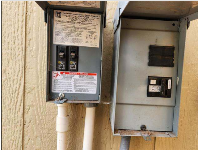
4.1 Item 5(Picture) rear exterior electrical panels
