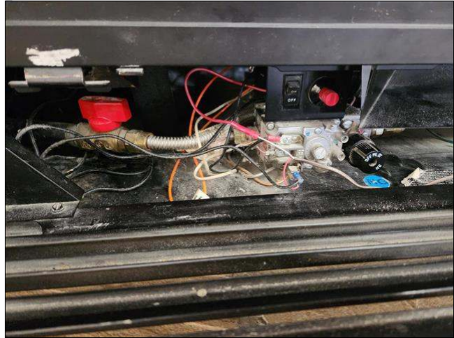
11.0 Item 2(Picture) fireplace gas valve
