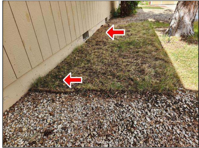
1.7 Item 2(Picture) negative grade at north side
