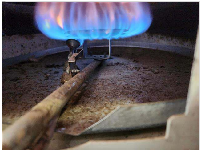
5.4 Item 2(Picture) water heater burner compartment
