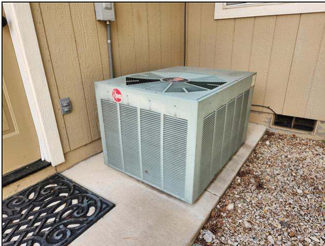
10.5 Item 1(Picture) condensing unit
