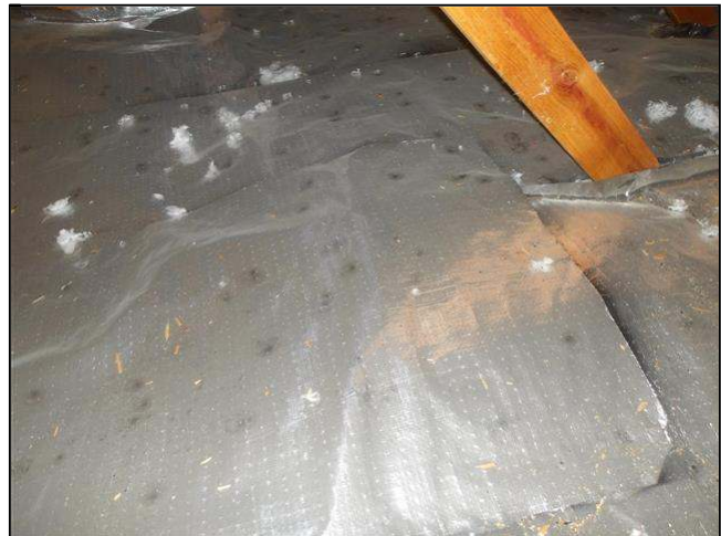
9.3 Item 2(Picture) drip stains from condensation
