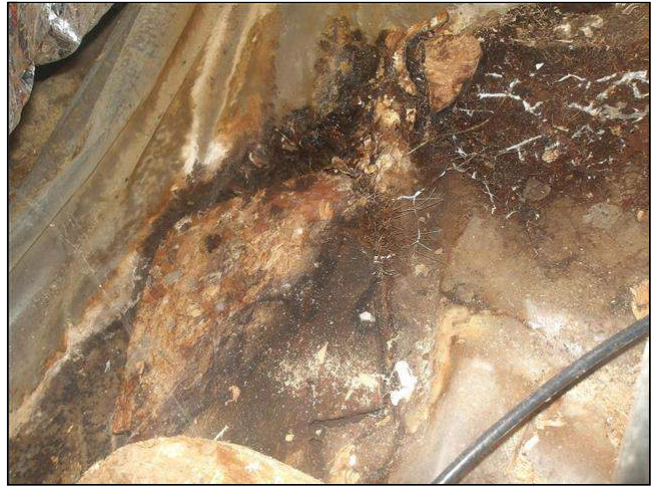
3.6 Item 4(Picture) moisture from leak
