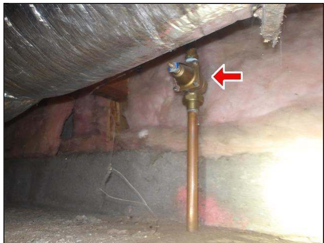
5.2 Item 2(Picture) Pressure regulator noted at the North side of crawlspace area
