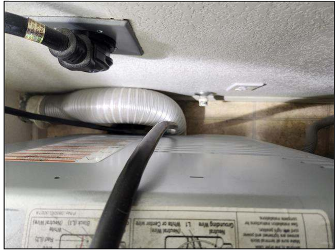
5.6 Item 2(Picture) laundry hook-ups
