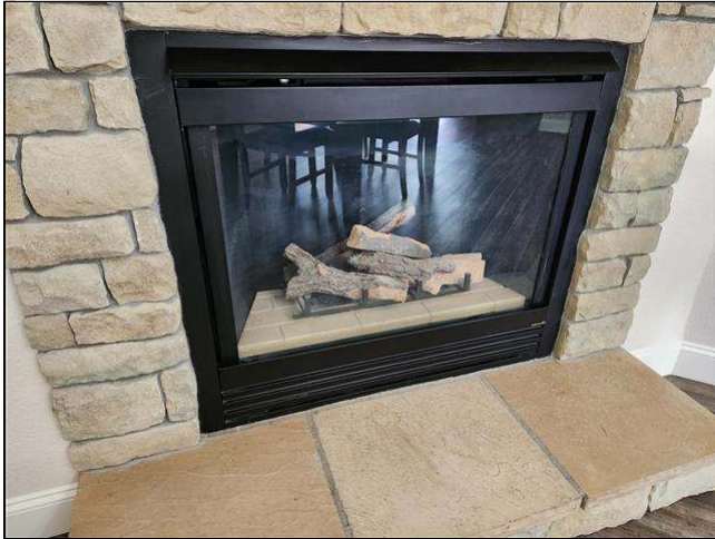
11.0 Item 1(Picture) living room gaslog fireplace
