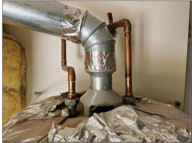
5.4 Item 4(Picture) water heater connections
