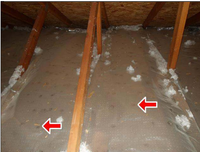
9.3 Item 1(Picture) drip stains from condensation
