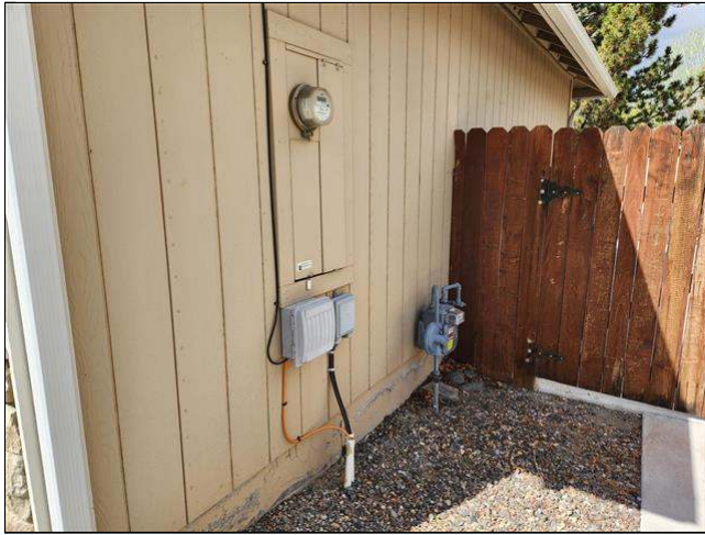
4.1 Item 3(Picture) main electrical panel
