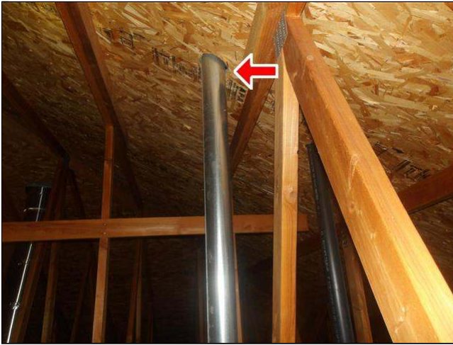
9.4 Item 1(Picture) properly ducted to the exterior
