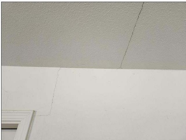
8.2 Item 1(Picture) typical settlement cracks
