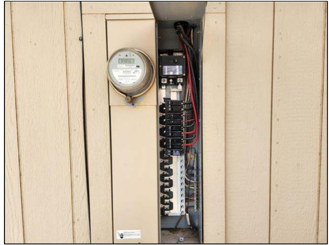
4.1 Item 4(Picture) panel conductors
