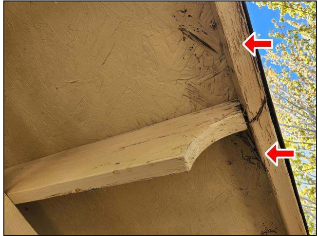
2.1 Item 2(Picture) Signs of past moisture intrusion were noted
