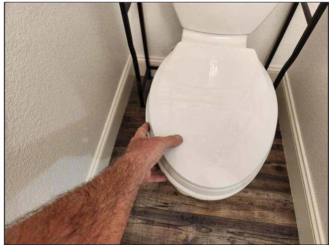
5.5 Item 2(Picture) toilet is loose at floor at the Guest Bathroom
