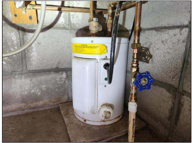
5.2 Item 4(Picture) Exterior kitchen plumbing
