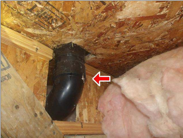
3.6 Item 1(Picture) floor joist top cord (and webbing) has been cut through
