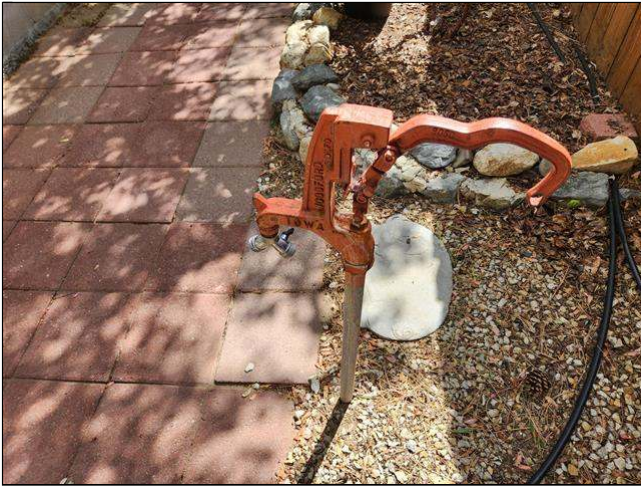
5.1 Item 1(Picture) non-operational at time of inspection
