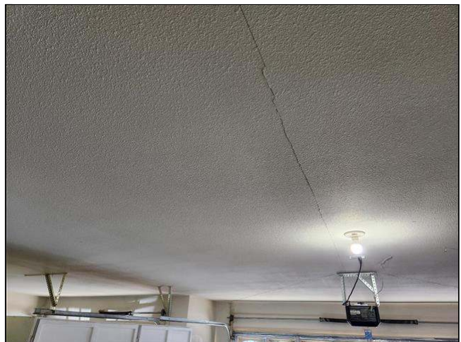
8.2 Item 2(Picture) typical settlement cracks
