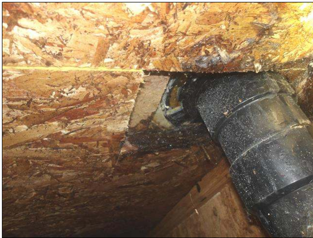
5.5 Item 1(Picture) saturated plywood subfloor from leak
