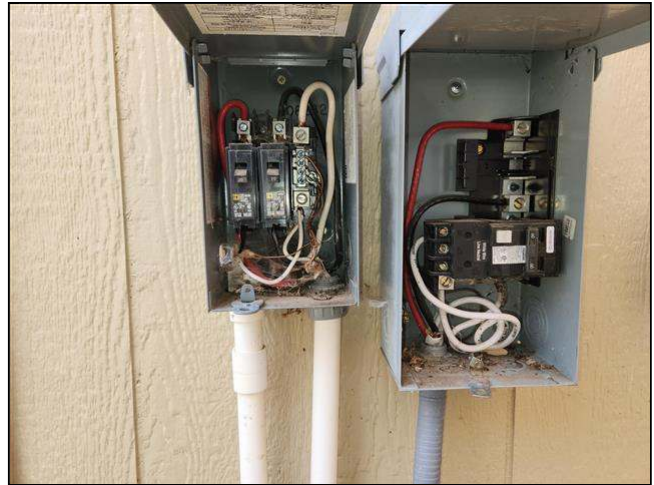
4.1 Item 6(Picture) panel conductors
