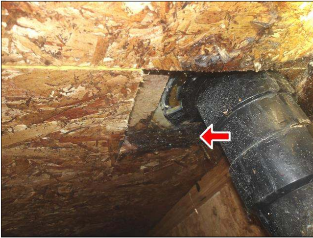
3.6 Item 3(Picture) saturated from a leaking toilet wax seal
