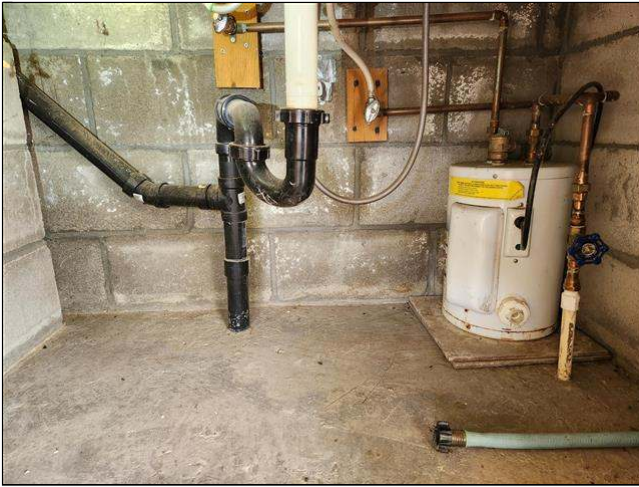
5.2 Item 3(Picture) Exterior kitchen plumbing
