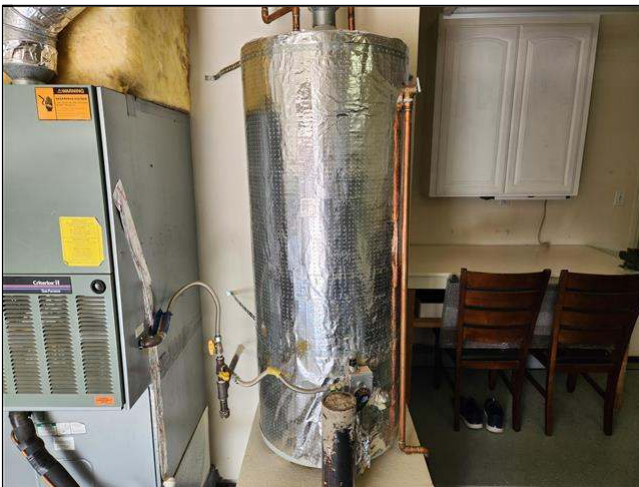
5.4 Item 1(Picture) water heater
