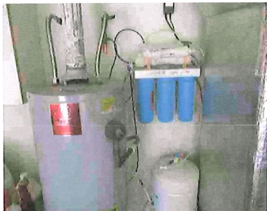
MECHANICALS AT GARAGE
