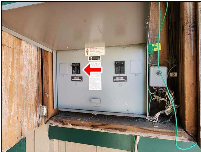
4.1 Item 1(Picture) main electrical disconnect
