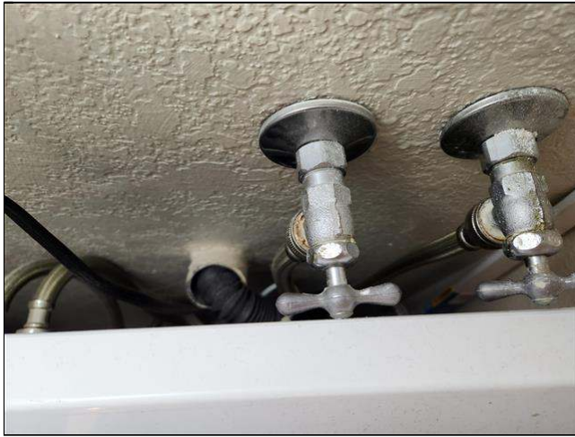
5.6 Item 1(Picture) laundry hook-ups
