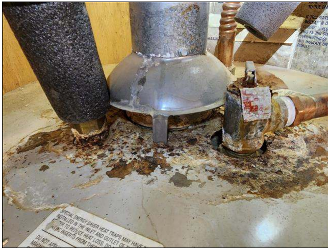
5.4 Item 3(Picture) past moisture leak at water heater
