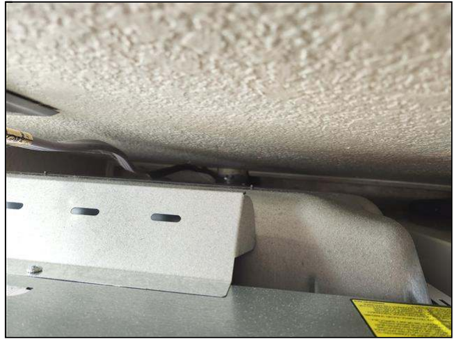
5.6 Item 2(Picture) laundry hook-ups
