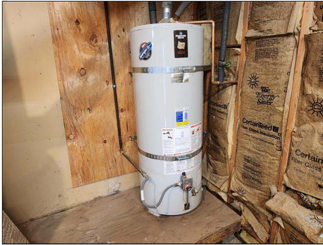
5.4 Item 1(Picture) water heater
