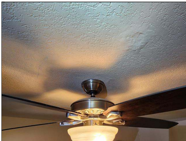
7.1 Item 1(Picture) master bedroom ceiling
