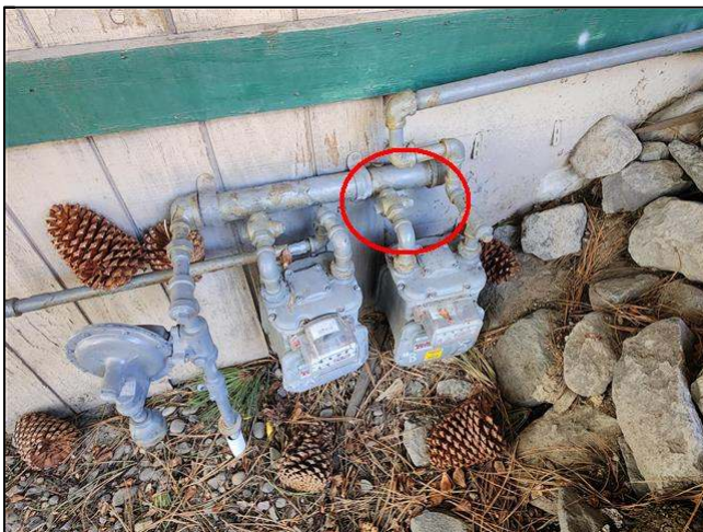
5.11 Item 1(Picture) main fuel shut-off valve
