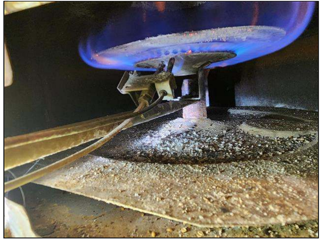
5.4 Item 2(Picture) water heater burner compartment
