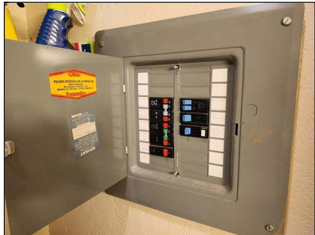
4.1 Item 2(Picture) laundry room panel
