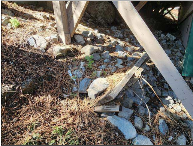
1.8 Item 1(Picture) failing retaining wall
