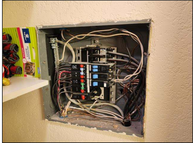
4.4 Item 2(Picture) laundry room panel
