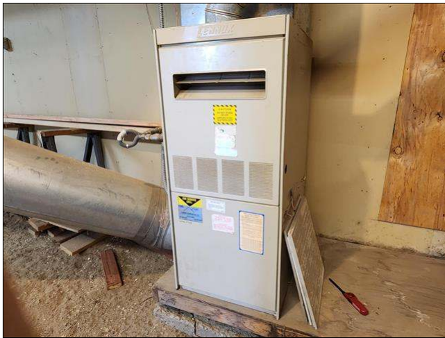
9.0 Item 1(Picture) forced air furnace
