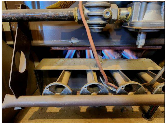
9.0 Item 2(Picture) furnace burners
