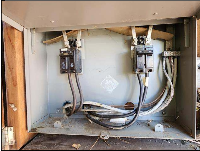
4.4 Item 1(Picture) main panel conductors
