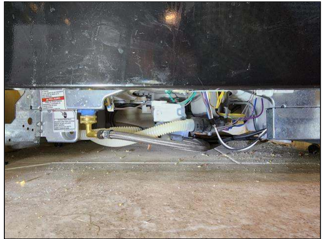
6.0 Item 2(Picture) dishwasher hook-ups
