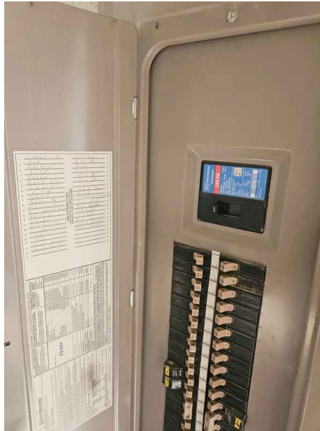
Service Entrance Conductors: Main Shut Off Location Garage Panel
