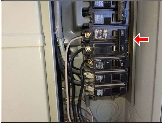
4.4 Item 1(Picture) 60 amp breaker, 30 amp wire
