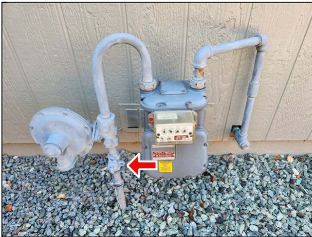
5.11 Item 1(Picture) main fuel shut-off valve
