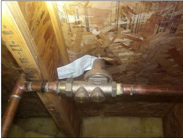
5.2 Item 1(Picture) pressure regulator in crawlspace
