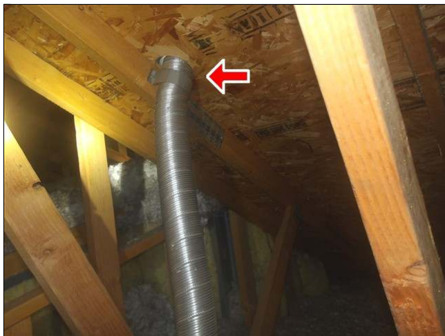
9.4 Item 1(Picture) properly ducted to the exterior
