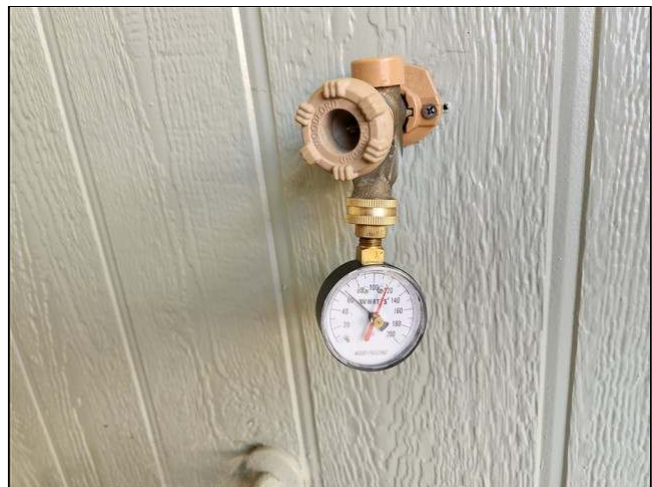
5.2 Item 4(Picture) water pressure at rear hose bib
