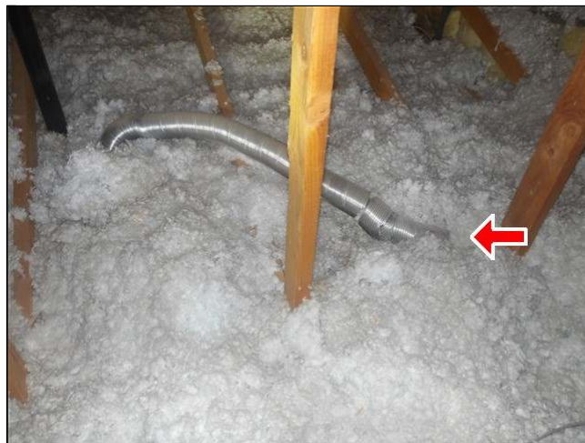
9.4 Item 2(Picture) does not vent to outside at the master bath
