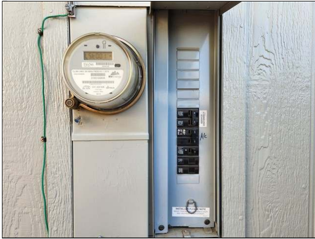
4.1 Item 3(Picture) main electrical panel
