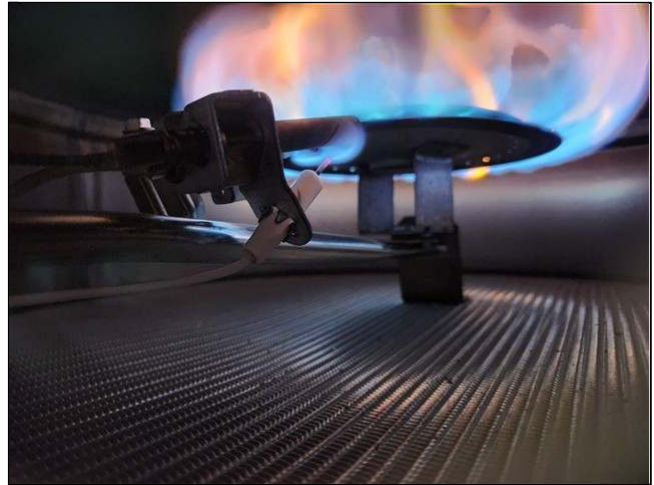
5.4 Item 2(Picture) water heater burner compartment
