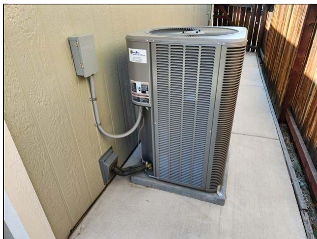
10.5 Item 1(Picture) condensing unit
