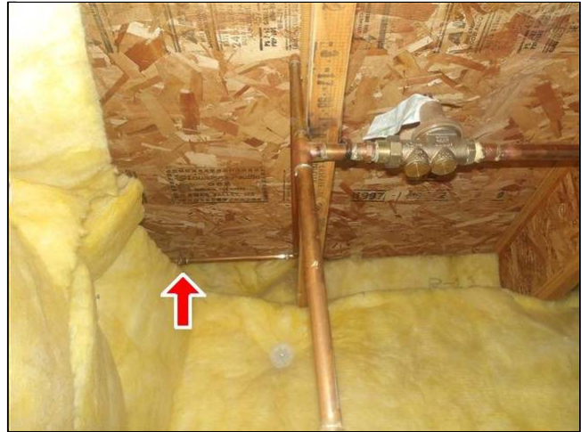
5.2 Item 2(Picture) north hose bib is before the pressure regulator
