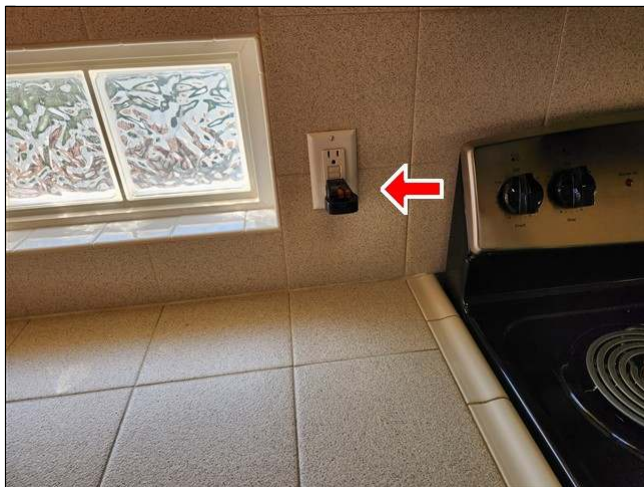
4.7 Item 1(Picture) defective GFCI at kitchen
