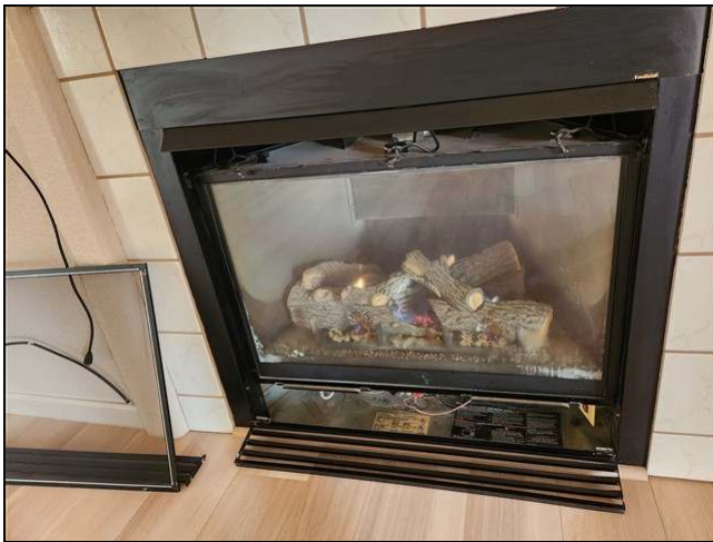
11.0 Item 1(Picture) Fireplace unit in Living room
