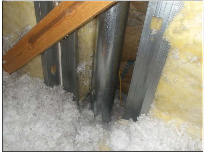
11.1 Item 2(Picture) proper clearances from combustible materials
