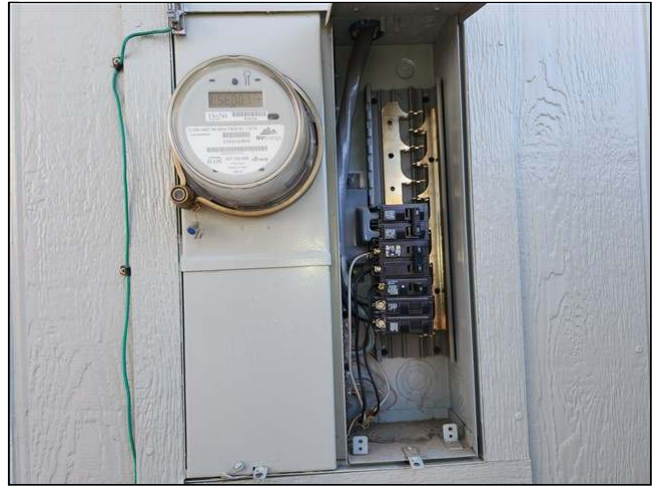
4.1 Item 4(Picture) main panel conductors
