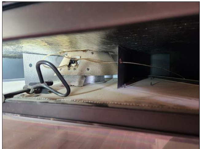
11.0 Item 4(Picture) Fireplace unit in Living room
