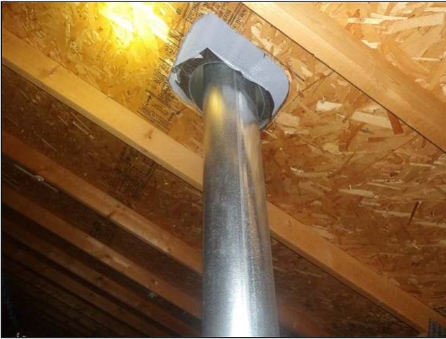
11.1 Item 1(Picture) proper clearances from combustible materials
