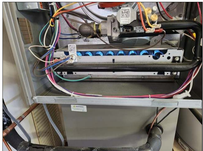
10.0 Item 2(Picture) furnace burners
