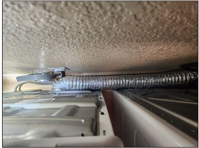
5.6 Item 2(Picture) Washer and dryer hook-ups
