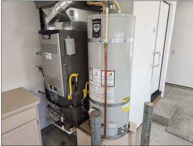
5.4 Item 1(Picture) water heater
