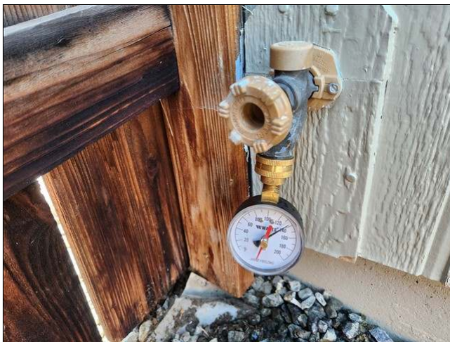
5.2 Item 3(Picture) water pressure at north hose bib
