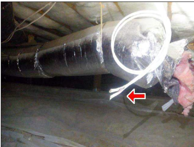
4.5 Item 2(Picture) loose end wires in crawlspace
