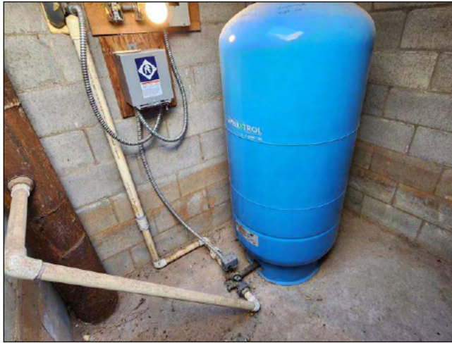
5.1 Item 1(Picture) well pump equipment
