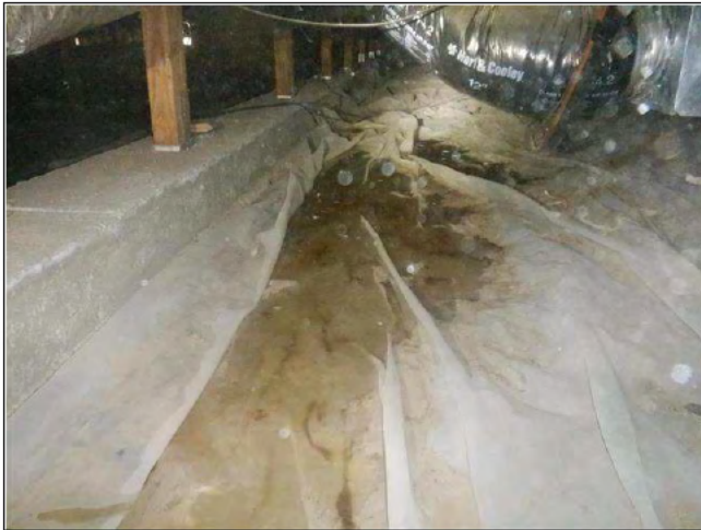
10.0 Item 5(Picture) pooled moisture in crawlspace
