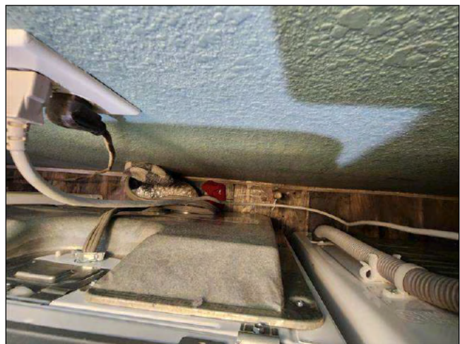
5.5 Item 2(Picture) laundry hook-ups
