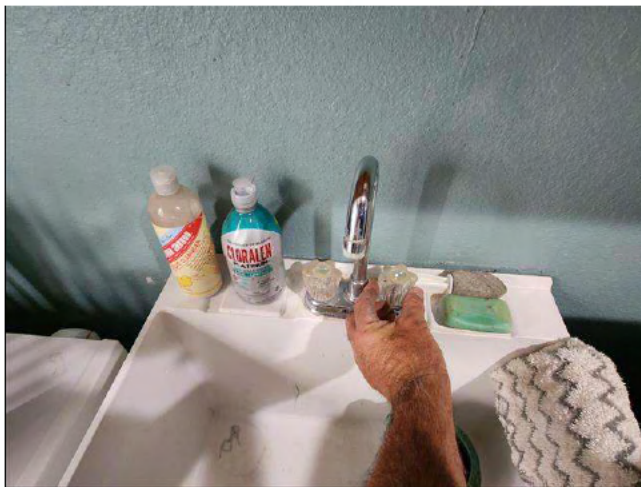
5.1 Item 7(Picture) no cold water supply at laundry sink
