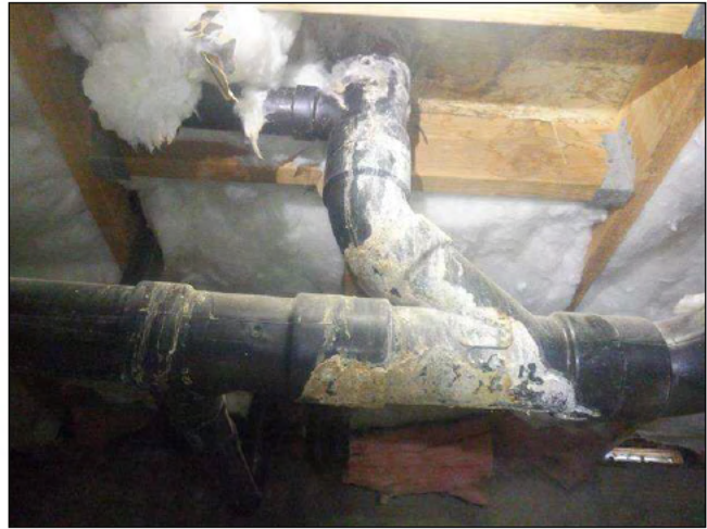
5.4 Item 3(Picture) signs of leakage under toilet
