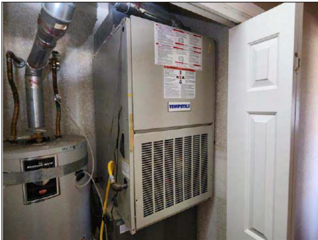
10.0 Item 1(Picture) forced air furnace
