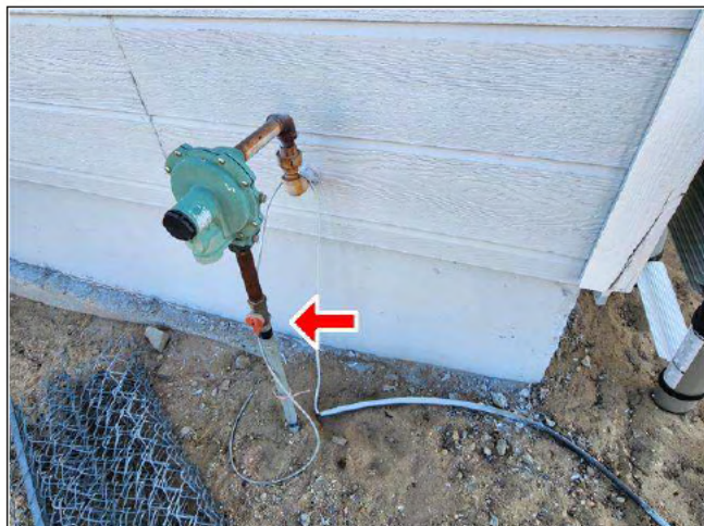
5.10 Item 1(Picture) main fuel shut-off valve
