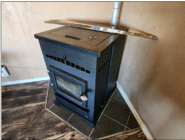
11.3 Item 1(Picture) living room pellet stove
