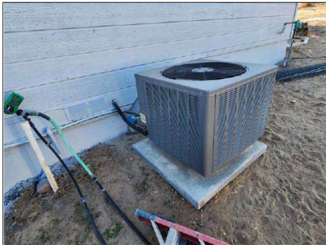
10.5 Item 1(Picture) condensing unit
