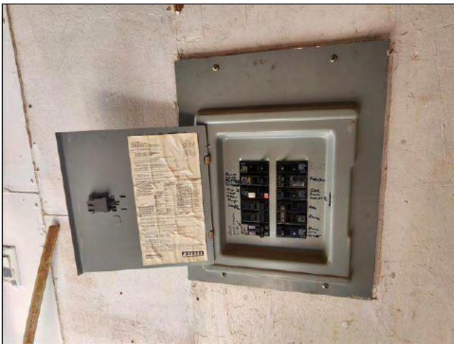
8.1 Item 1(Picture) garage panel
