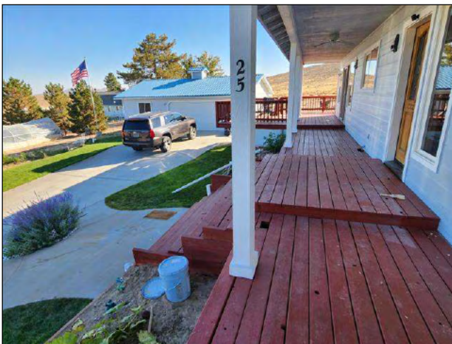
1.6 Item 1(Picture) missing handrails at steps
