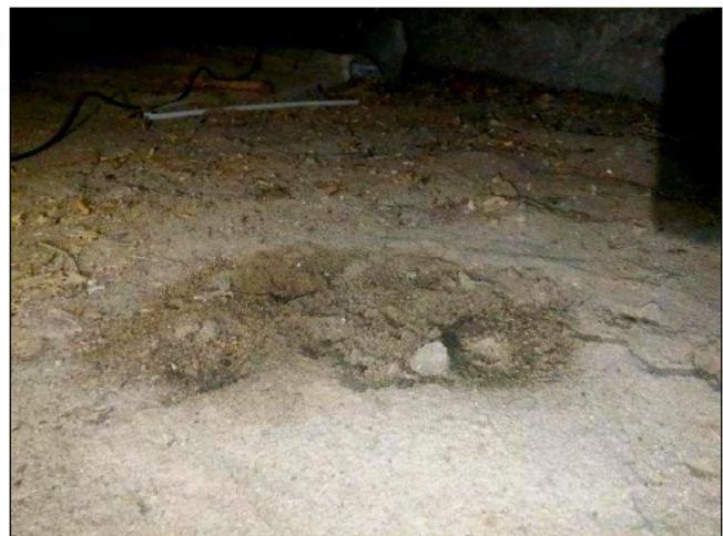
5.2 Item 2(Picture) moisture from leak
