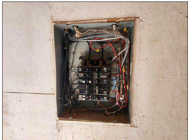
8.1 Item 2(Picture) garage panel conductors
