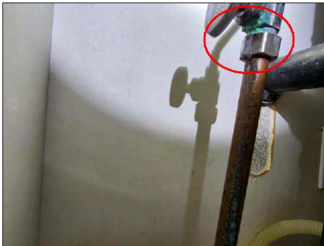
5.1 Item 3(Picture) hot water supply shut-off valve
