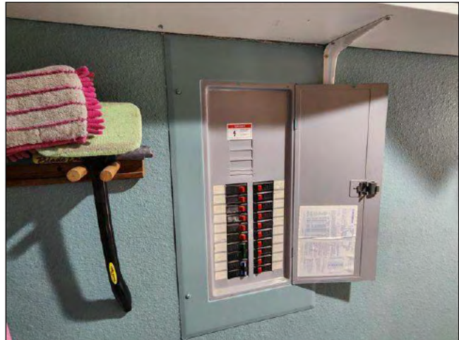
4.1 Item 2(Picture) laundry room panel
