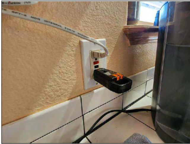
4.7 Item 1(Picture) faulty GFCI at kitchen
