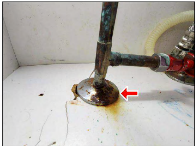
5.1 Item 4(Picture) moisture from leak
