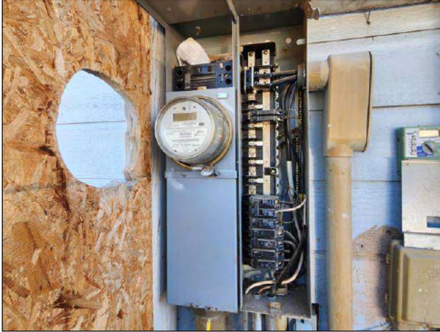
4.4 Item 1(Picture) main panel conductors
