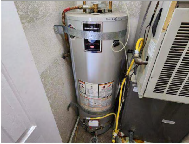
5.3 Item 1(Picture) water heater
