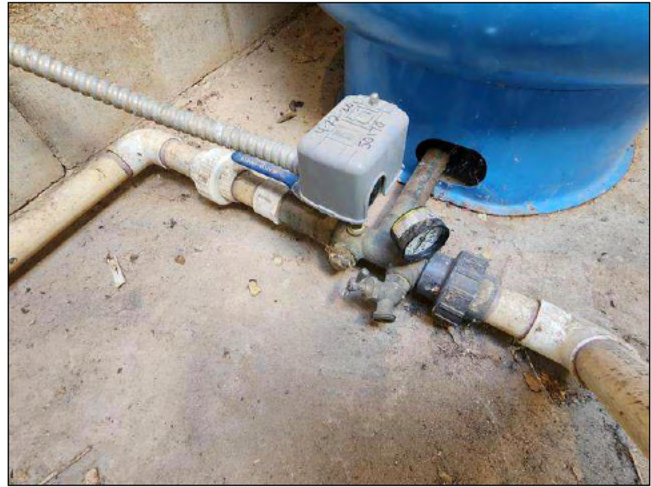
5.1 Item 2(Picture) well pump equipment
