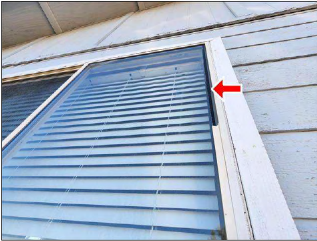
1.4 Item 1(Picture) missing exterior dust seals
