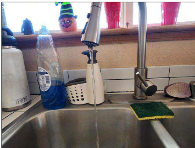
5.1 Item 5(Picture) low volume at hot side
