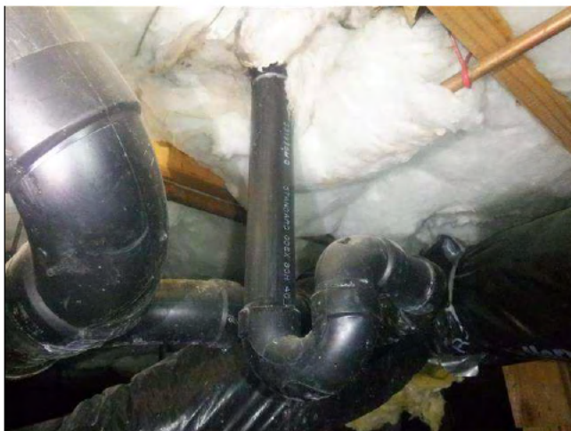
5.2 Item 1(Picture) guest bathroom shower drain
