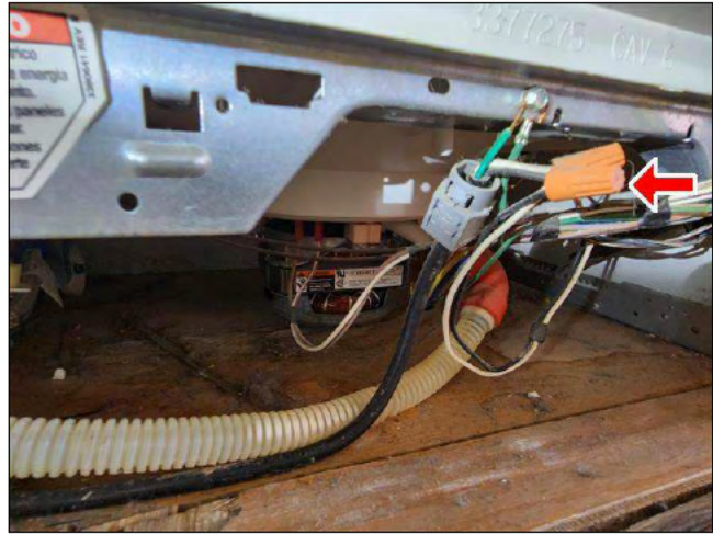
6.1 Item 2(Picture) open electrical connection under dishwasher
