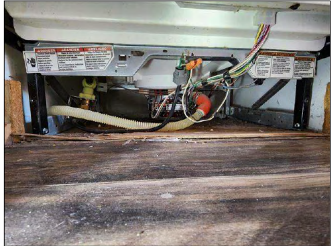
6.0 Item 2(Picture) dishwasher hook-ups
