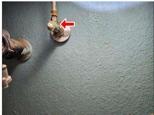
5.1 Item 8(Picture) supply valve missing handle
