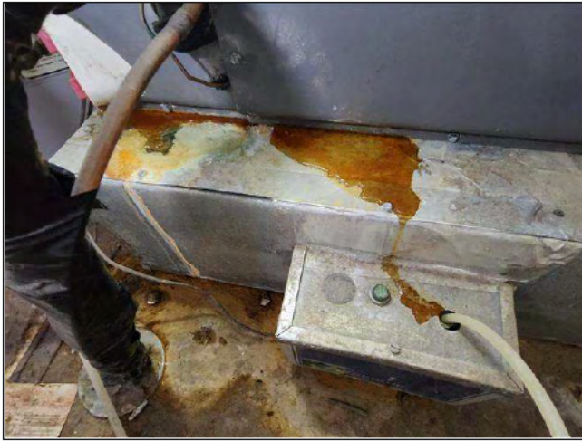
10.0 Item 3(Picture) moisture from furnace
