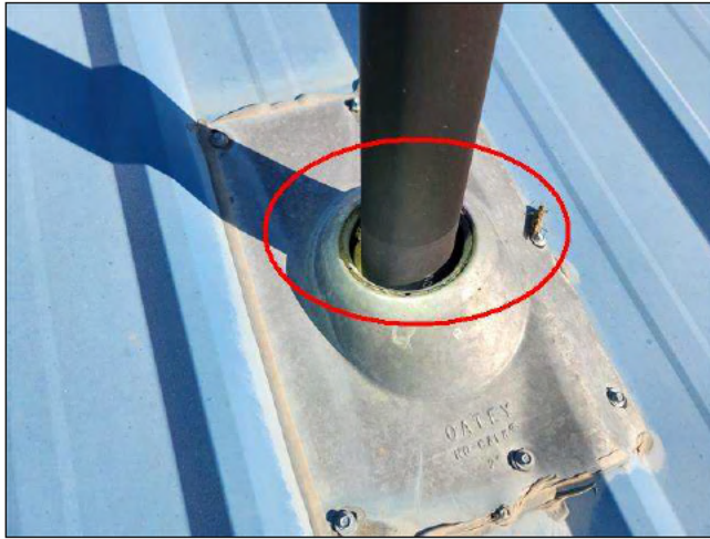
2.3 Item 1(Picture) plumbing vent pipe seals
