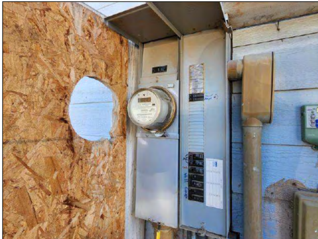
4.1 Item 1(Picture) main electrical panel
