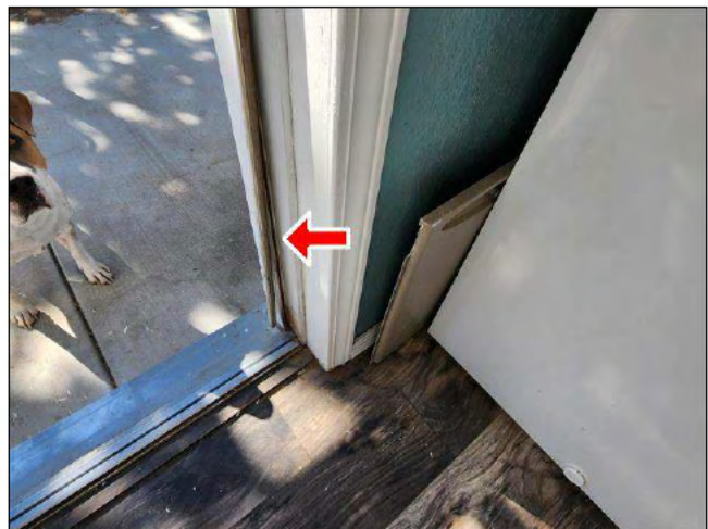
1.3 Item 2(Picture) weather stripping at laundry door
