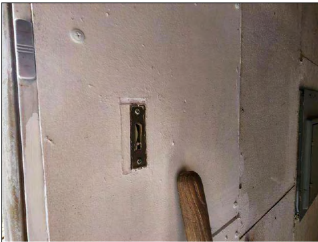
8.9 Item 1(Picture) broken control button
