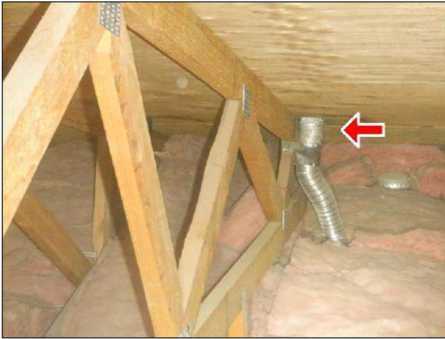
9.4 Item 1(Picture) properly vented to exterior
