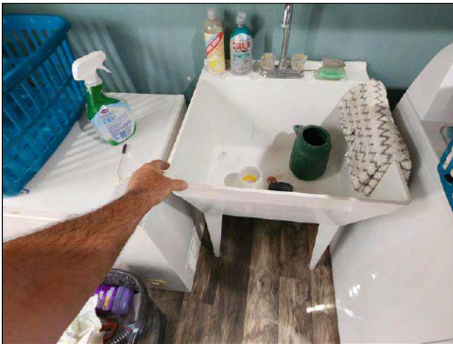
5.4 Item 1(Picture) secure laundry sink
