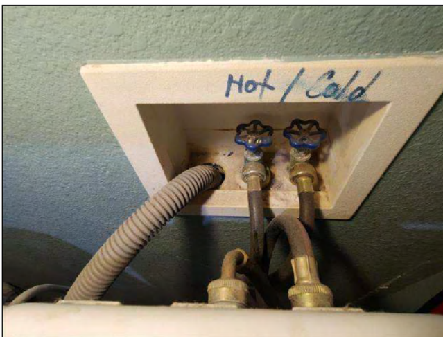
5.5 Item 1(Picture) laundry hook-ups
