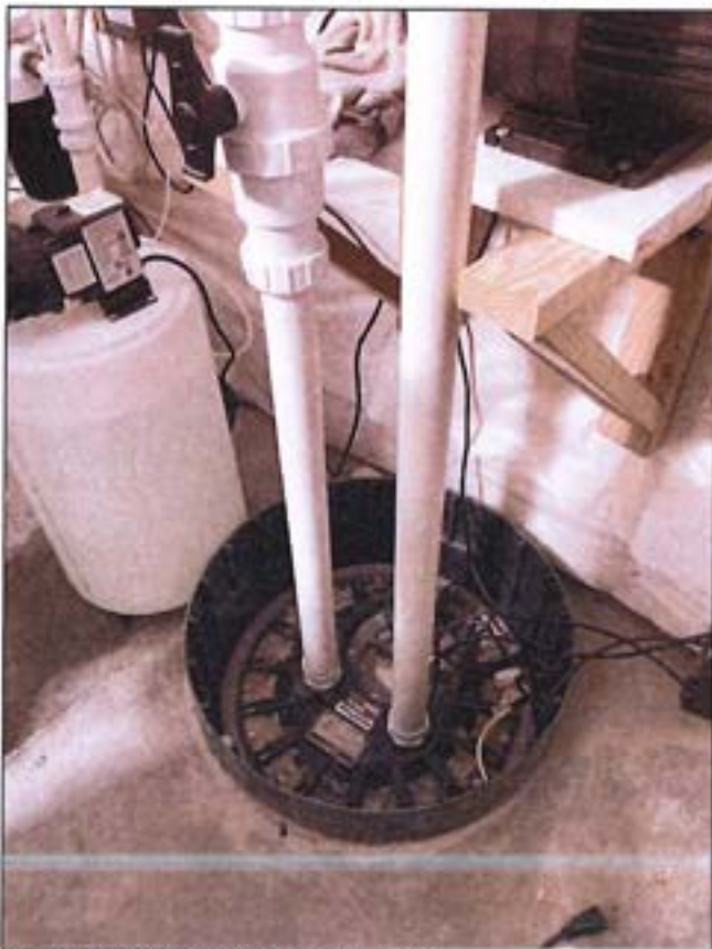
6.6 Item 1(Picture) sewage pump
