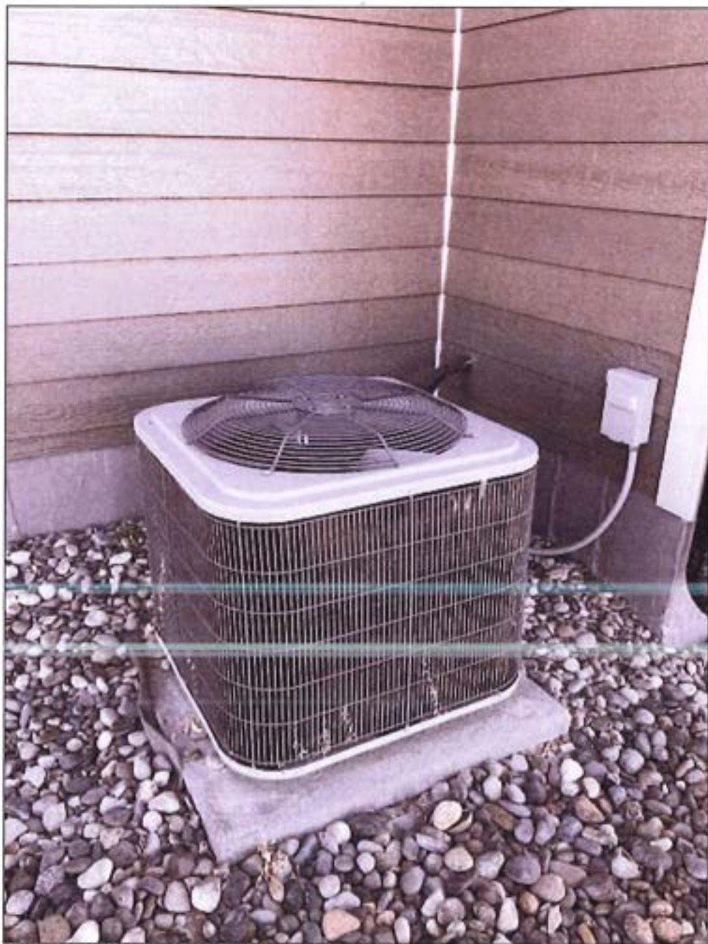
8.8 Item 1(Picture) Clean cooling fins as needed.
