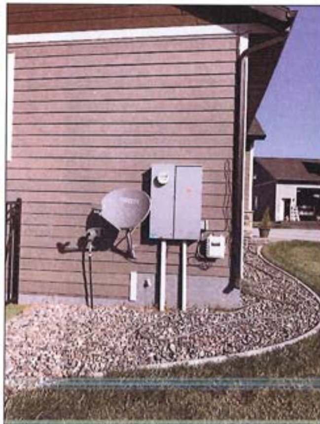
7.6 Item 2(Picture) service disconnect
