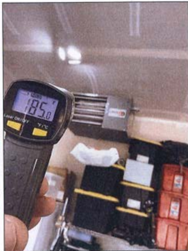
8.0 Item 5(Picture) garage: 185 F after running 2 minutes
