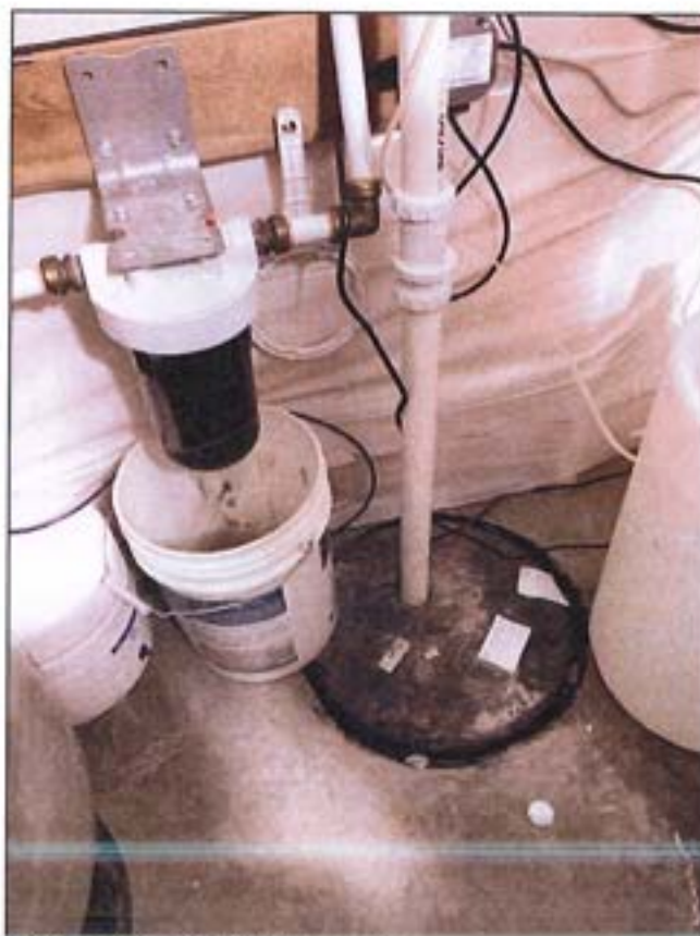
6.6 Item 2(Picture) sump pump
