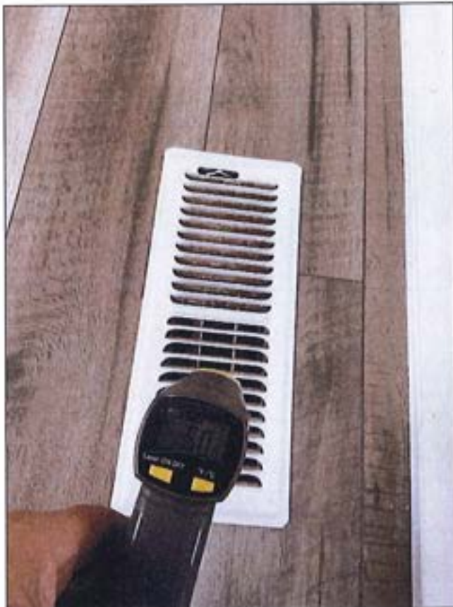
8.8 Item 3(Picture) Ac temp was 50 F after running 5 minutes
